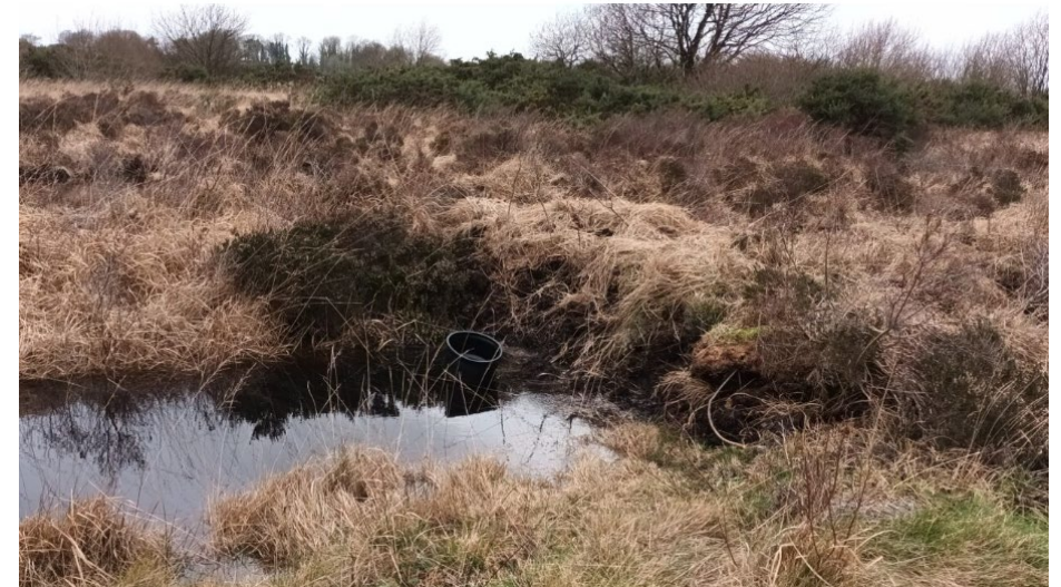
A pipe through a peat dam was installed to give flexibility to the farmer if they wished to adjust the water levels within the drain on a farm in Co. Roscommon. (Source: FarmPEAT)
