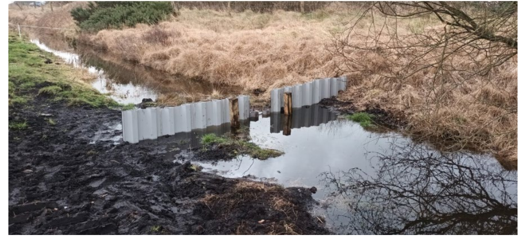
Drain on a farm in Ireland with plastic dam was installed – re-wetting agricultural peat land. (Source: FarmPEAT)
