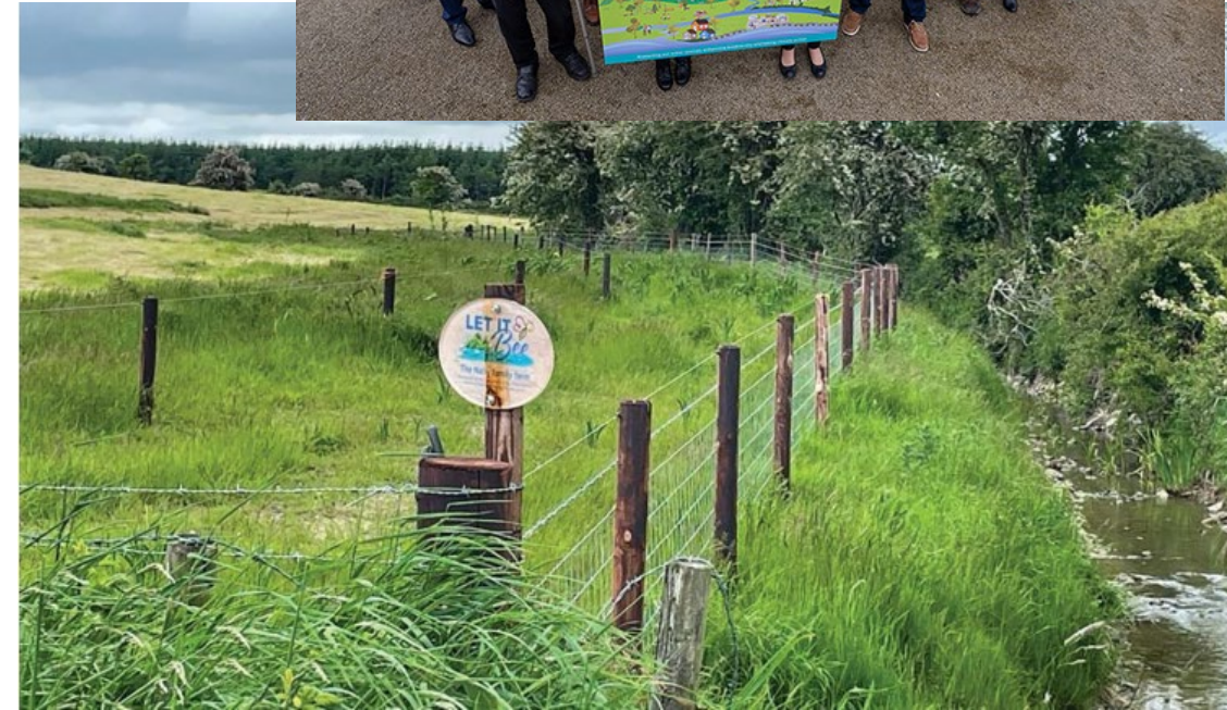
Fencing erected as part of source protection works in Irish Group Water Scheme (from: NFGWS -Source-Protection-Phase-II-Report).
