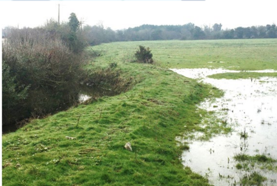
A low earthen bund or bank reducing or preventing overland flow entering the watercourse (NFGWS, 2020)
